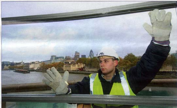
GLASS ACT: Killby & Gayford is carrying out a £200,000 refurbishment of the Tower Bridge Exhibition Centre ticket office for the City of London. The new look incorporates modifications to the glazed façade. The works will take place over a 12-week period. Photograph: Mike O'Dwyer
